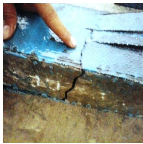
Figure 5. Failure of Three sided continuous CFRP wrapped beam.(7 days)
