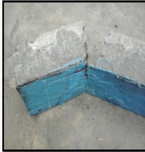
Figure 3. Failure of one sided CFRP.(7 days)
