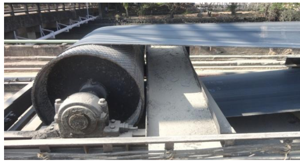
Figure 2.1. Corrosions affected drum
