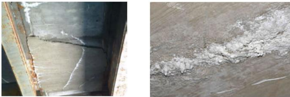
Fig6. Leached salts and minerals on concrete external (Zoran Bonić, Gordana Topličić Ćurčić, et al. 2015).
