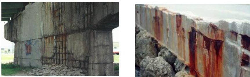
Fig8. Reinforcement erosion of the construction sections in contact with soil (Zoran Bonić, Gordana Topličić Ćurčić, et al. 2015).
