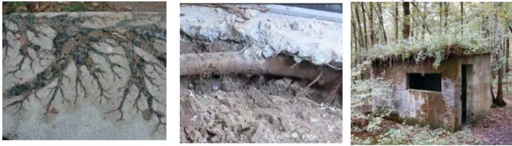
Fig2. Deprivation of concrete triggered by the tree roots and flora (Zoran Bonić, Gordana Topličić Ćurčić, et al. 2015).
